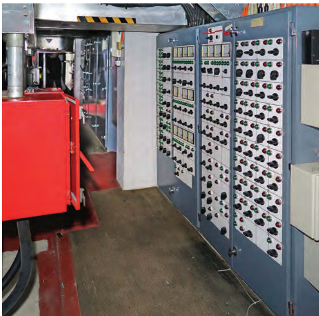
The electrical plant room on the top floor.
